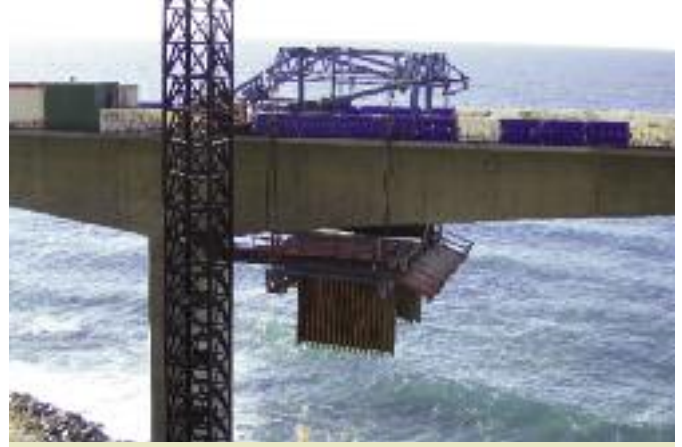
After completion of cantilevering, the travellers were "back launched" to the pier for disassembly and relocation to the next piers.
