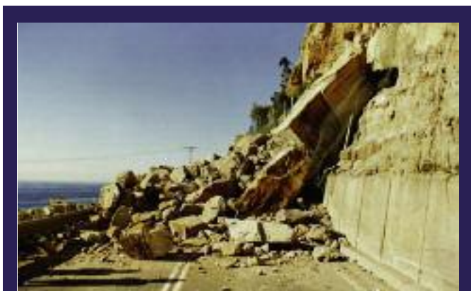
Rock falls and embankment failure had been very regular over the lifespan of the road, with over 50 rock falls reported between 1996 and 2003. The road was finally closed in 2003 after major cracks up to 1m wide developed.
