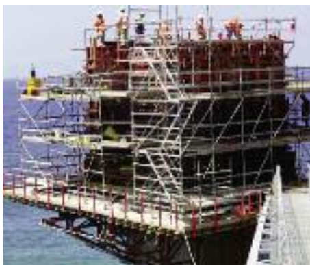
A large 15.4m by 12.5m four module working platform was attached to each pier to allow for construction.
