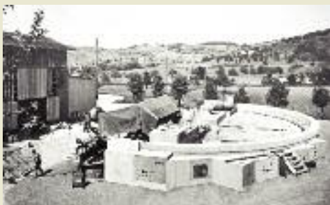
Full-scale grouting and replacement test with tendons consisting of 7mm diameter wires in tightly twisted groups of three wires each, as well as with tendons composed of strands.
