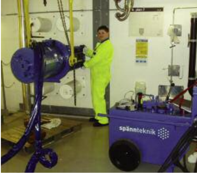
Periodical technical inspection of the tendons with lift-off tests at the Forsmark nuclear power plant in Sweden.
