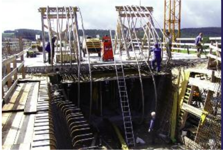
Section joint with BBR VT CONA CMI 1506 fixed couplers and overlapping prestressing tendons.
