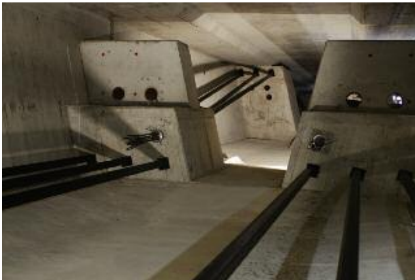
External prestressing tendons – in the foreground, span pilaster strip with curvatures and anchorages and, in the background, cross support with curvatures.
