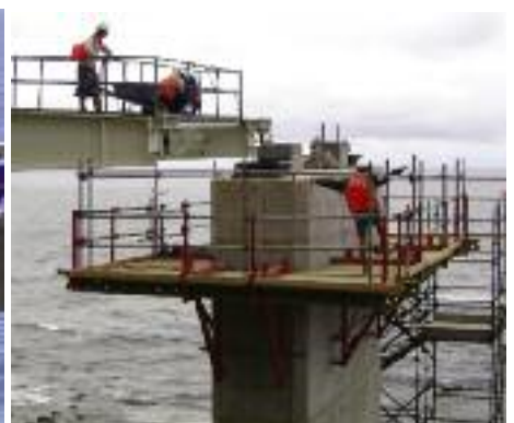
For incremental launching, a kinked 30t launch nose was fitted to reduce the bending moments and deflections.
