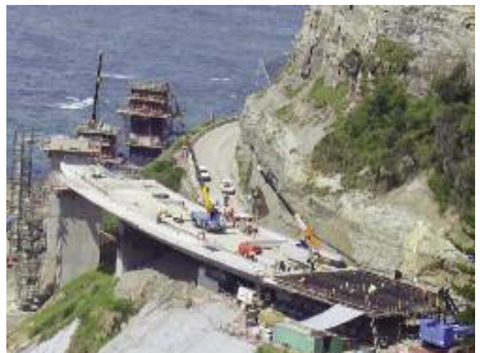
The incrementally launched bridge was constructed at the northern abutment and launched south over piers 1 through to 7.
