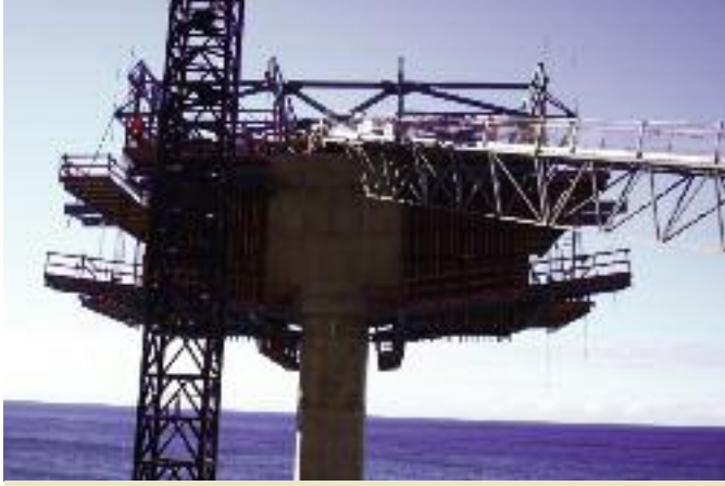
The travellers were assembled in a back-to-back pair arrangement on each completed pierhead for the first north and south segment pours.
