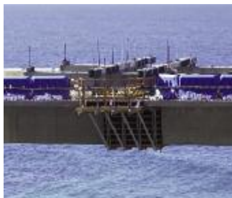
Closure pours utilised a series of additional systems – including a small travelling system and special formwork.
