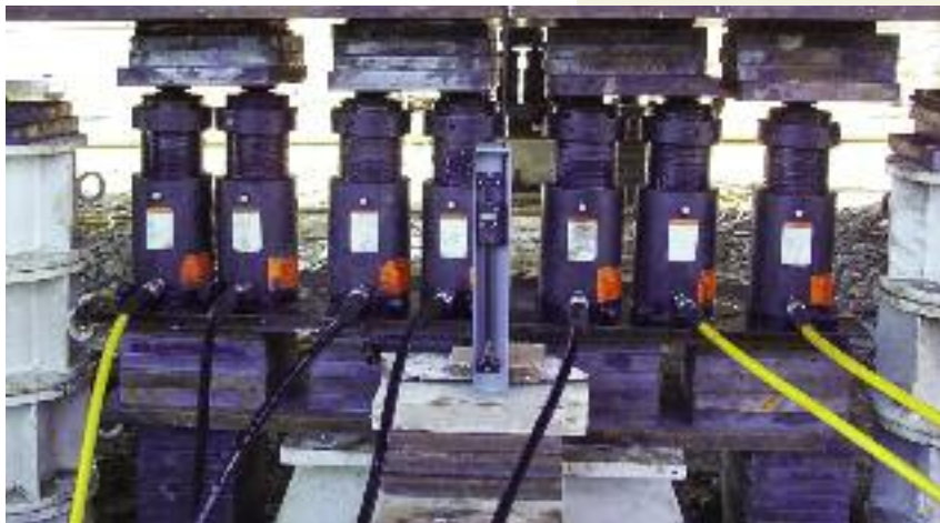
A patch loading test was done to assess the behaviour of the structure.
