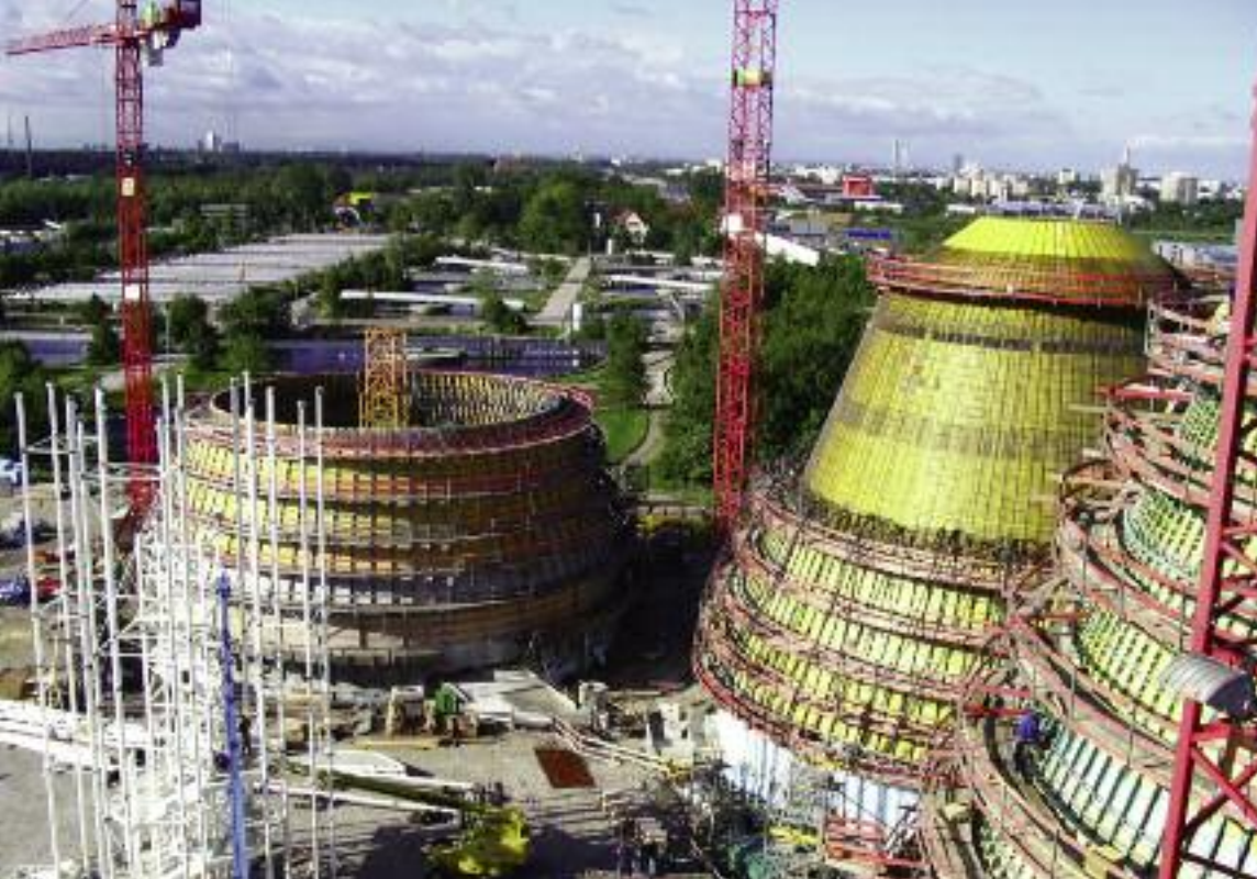
View of digestion tank 1 – construction stage 5 completed, digestion tank 2 – construction stage 5 completed, inner framework construction stage 9 completed, and part view of digestion tank 3 – construction stage 8 completed.
