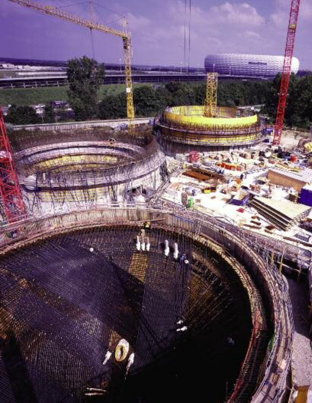
Overview of new digestion tank system – front left, digestion tank (DT1) with installed conic prestressing tendons, behind DT2 with inner funnel formwork before concreting, DT3 with rising inner formwork and, rear right, DT4 with circumferential funnel formwork.
